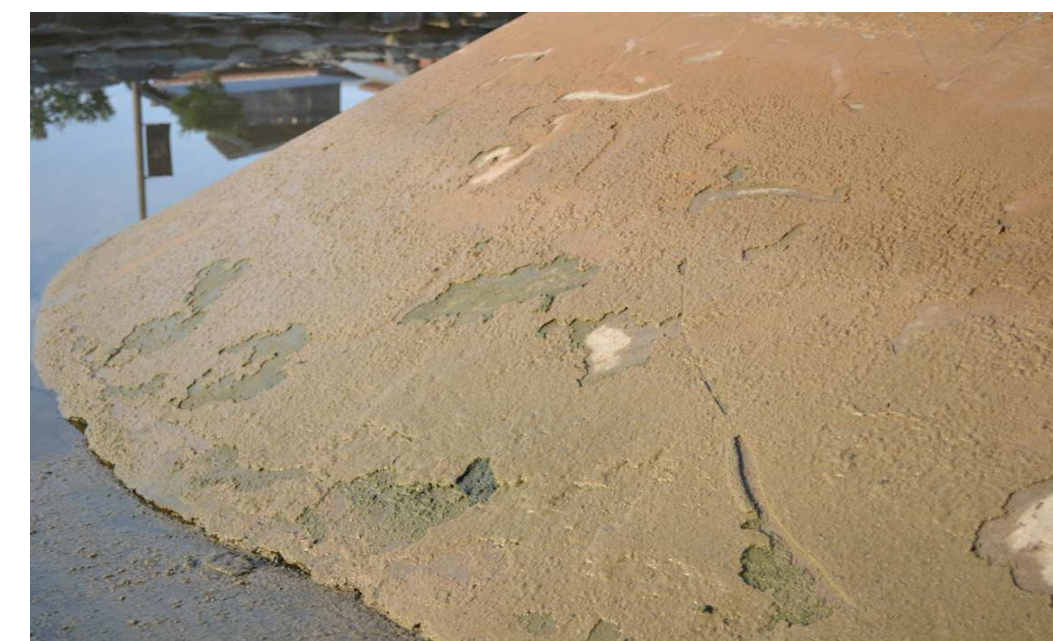
Heavy algal growth observed on concrete wall of boat loading ramp
